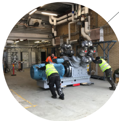
Gothenburg heat pumps
